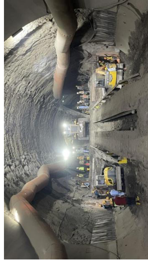
Figure 2. KCIC maintenance machinery equipped with generator and lighting group
