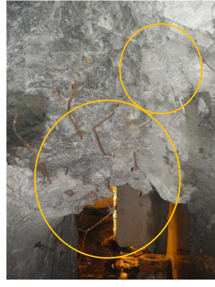
Gambar 10. Heavy Damage (Doc. UG Geotech & Hydrology)
