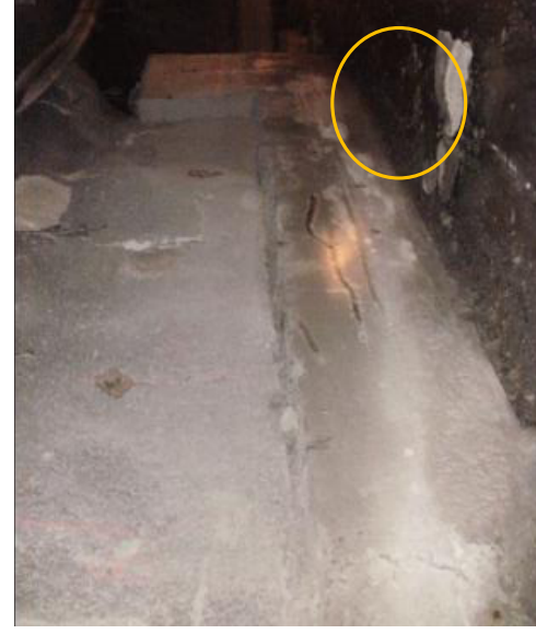
Gambar 9. Moderate Damage (Doc. UG Geotech & Hydrology)
